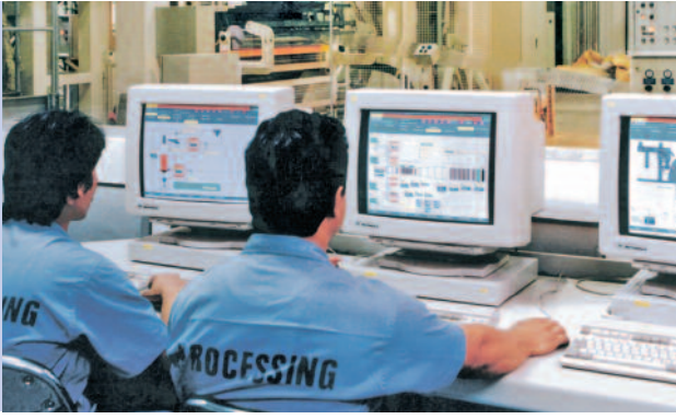
Process control system
